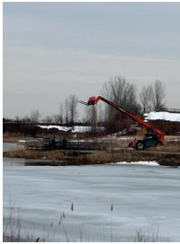
Picture of the work to stabilize and level the piers at Oneida Lake, for the Membership's and Community enjoyment and safety.
