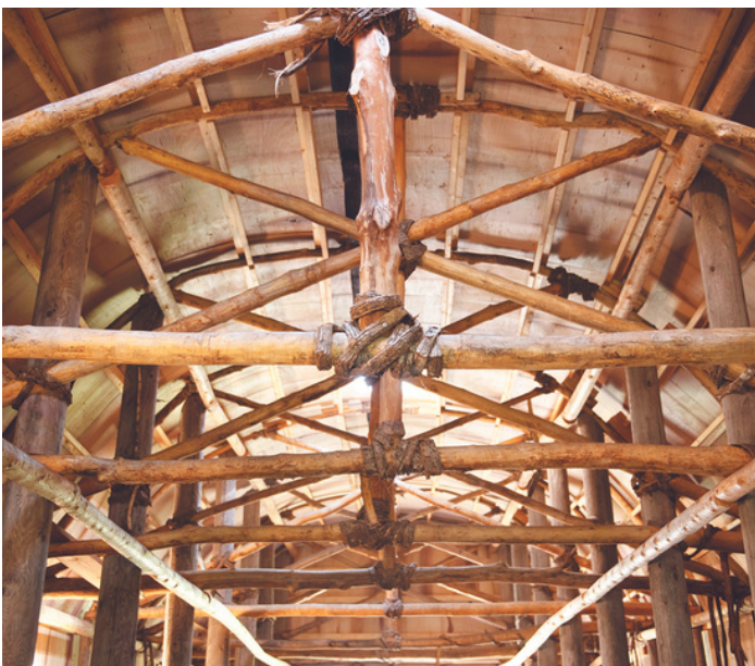
Photo: Inside of Longhouse
