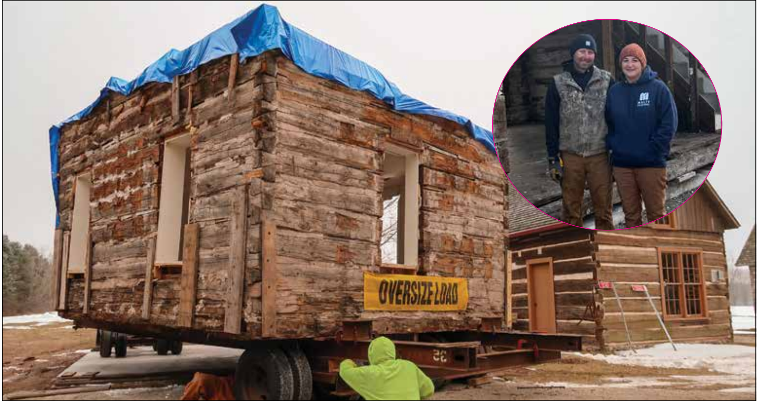
Charlie and Crystal Meltz, of Meltz Construction, in front of the donated Lee Gordon II and Pearl McLester log home originally located on County Line U after it was placed in it's new permanent home at the Amelia Cornelius Culture Park in January 2024. The log home will soon be refurbished to become another symbol of Oneida history, along with the 5 other log homes on display.
