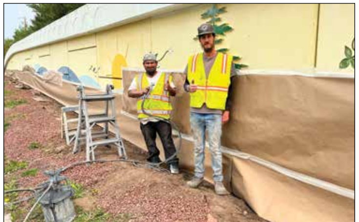
▲ Photo courtesy Michelle Danforth Anderson David Vera and Travis Fabian of Integrity Coaters, LLC bring color back to the faded retaining wall located on Hwy 54 near the VFW.
