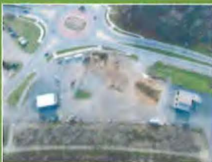
December Installing the new underground storage tanks at the new 54 One Stop
