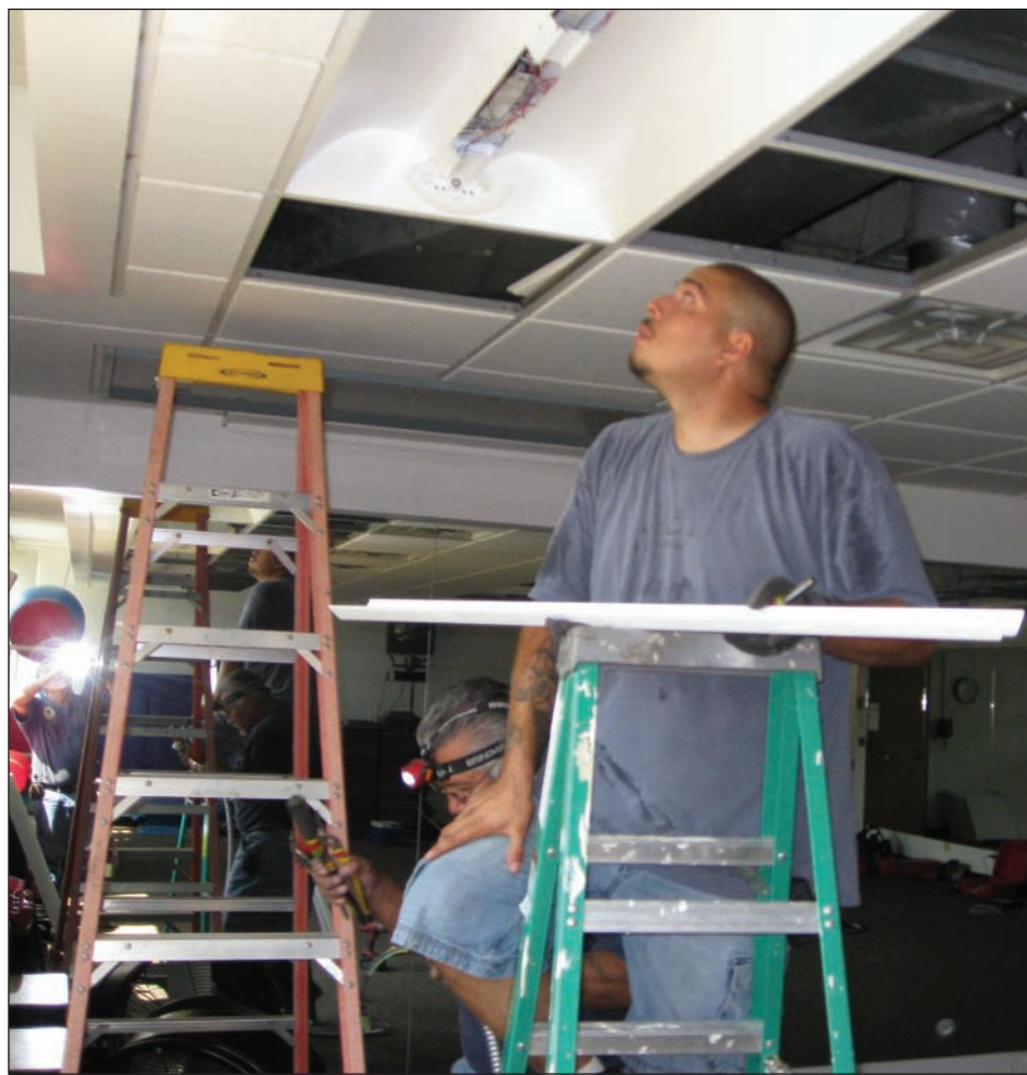
Photo courtesy of Oneida Department of Public Works Mitch Skenandore of the Oneida Department of Public Works replaces older lighting with new, more energy efficient lamps as part of at $324,700 stimulus block grant.
