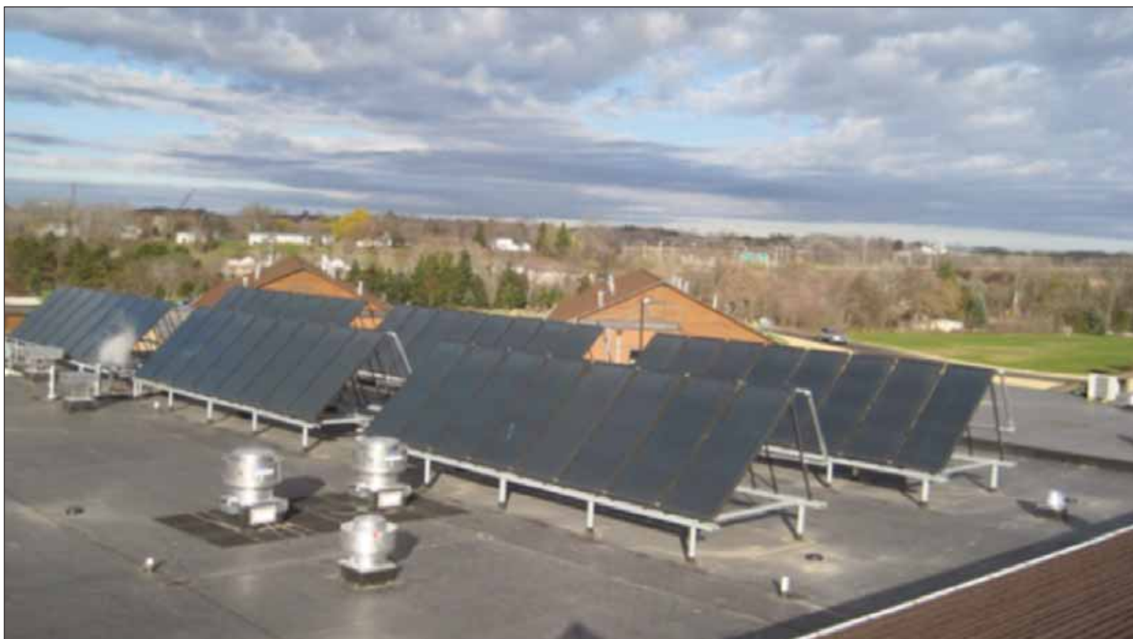
Submitted photo Solar hot water panels on AJRCCC.
