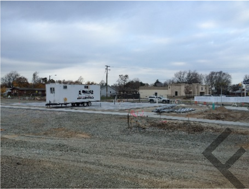
Construction Loan in progress – Future new home of Ridgeview Liquor on Ridge Rd in Green Bay (photo Nov 2015)
