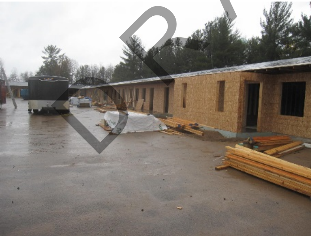
Construction Loan in progress – Rehab and expansion of an existing building on the Mole Lake Reservation (photo Oct 2015)
