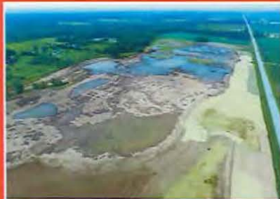
The view from 400' above Shady Dr. The site is available to the general public and can be used for canoeing, wildlife viewing, and hiking. NO hunting, fishing, or trapping during construction.
