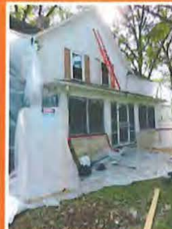
September EHSD assisted in the demolition of this house on Hwy 54 by managing the asbestos removal.
